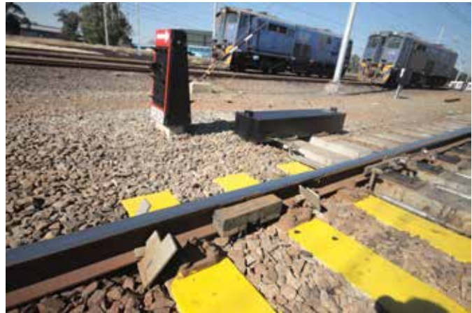
The basic elements of the yard control system: an axle-counter detection point, an indicator and a points machine.
