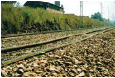
Figure 6: Vertical alignment defects.
