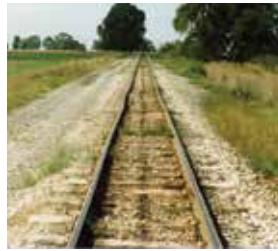
Figure 7: Horizontal alignment defects.
