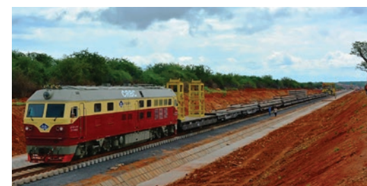
Construction of the Kenya Standard Gauge Railway (SGR). Photo: Kenya Railways - https://www.facebook.com/Kenya-Railways-248578828508174/
